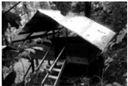
Above: the new sleeping shed at Afi base camp; below: the renovated communal shed at Afi base camp Photos: Inaoyom Imong
