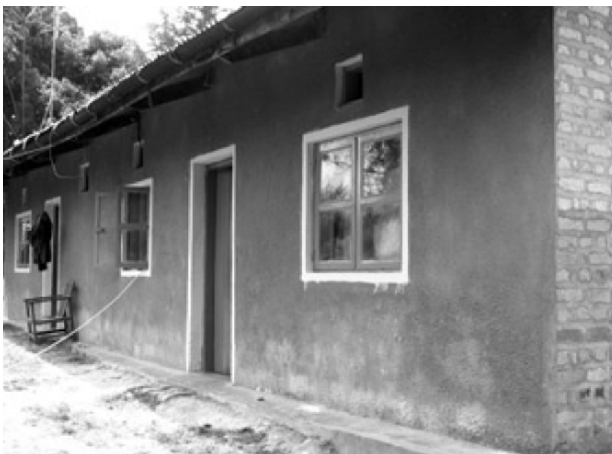
Front of the office of the Ruhija outpost: cracks were repaired, the ceiling painted, cover beads fixed, the splash apron repaired.
