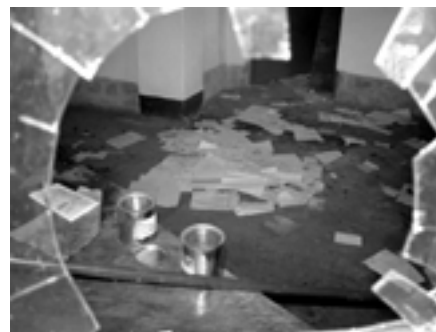
Destruction in the health center
