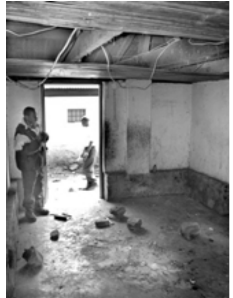
Destruction in a ranger house
